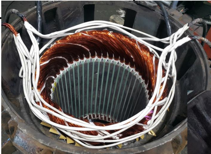
MOTOR 160KW 4P REWINDING
